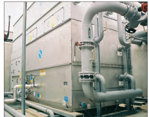
Intake and Discharge Sound Attenuation
