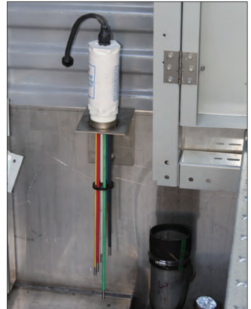
Electric Water Level Control
