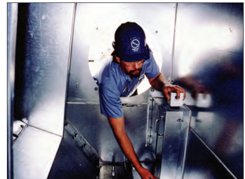
Mechanical Water Level Control Inspection
